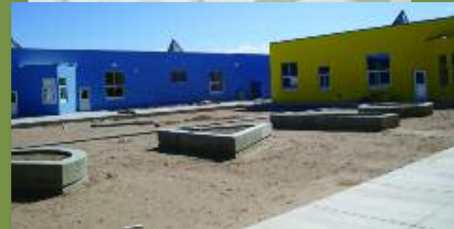
Helen Cordero Primary School will be LEED Silver certified and will include Ground Source Heat Pumps HVAC system.
